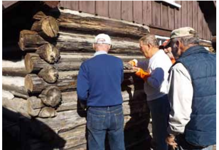
Dale Marsden and Rod fill cracks as Joe Larson and Bob Kolek look on. Joe and Bob prepared the wire and mortar.
